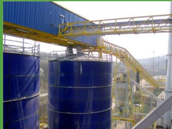
operational silos of wood chips in front of boiler room
