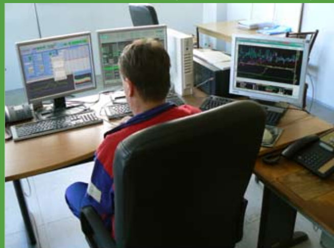
technological control room of the plant
