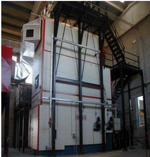
Photo: Biomass Boiler
