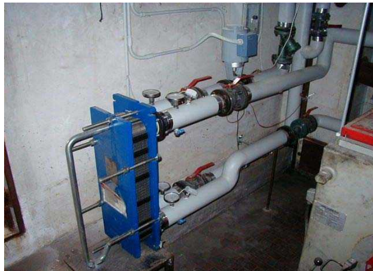
Photo: User heat exchanger
