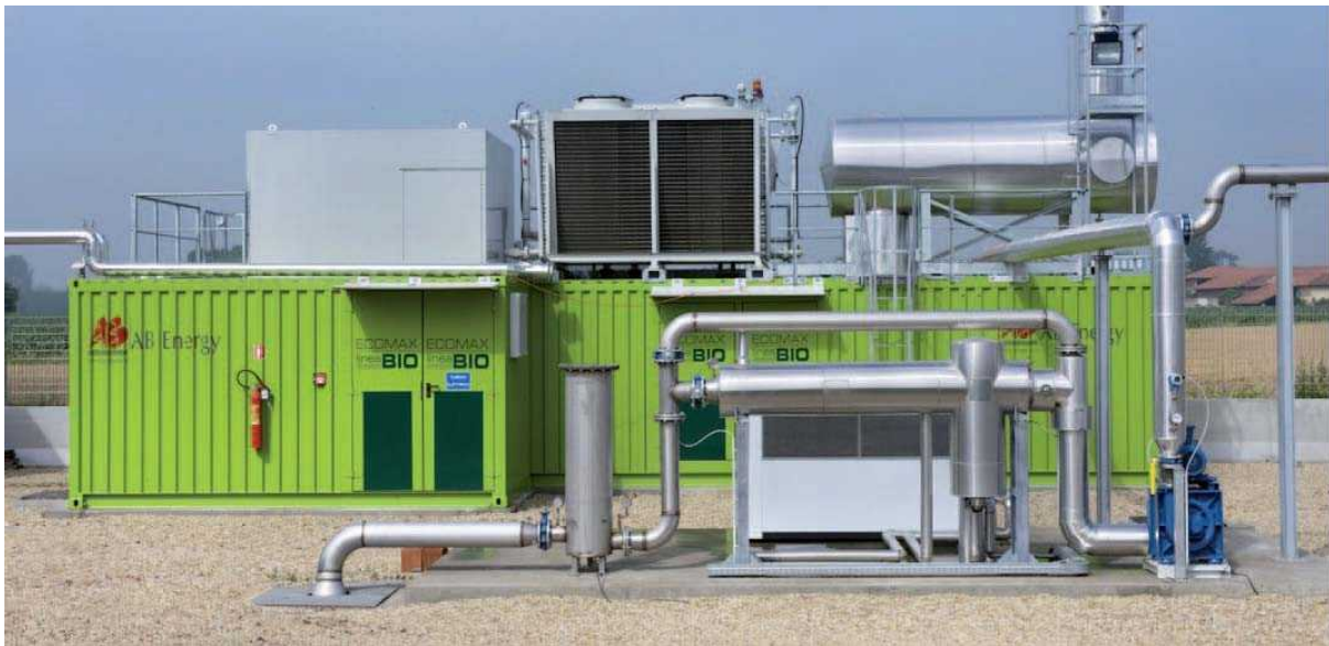
Photo: Jenbacher Gas Engine
