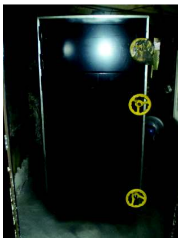
Pic.8 Small scale biomass boiler
