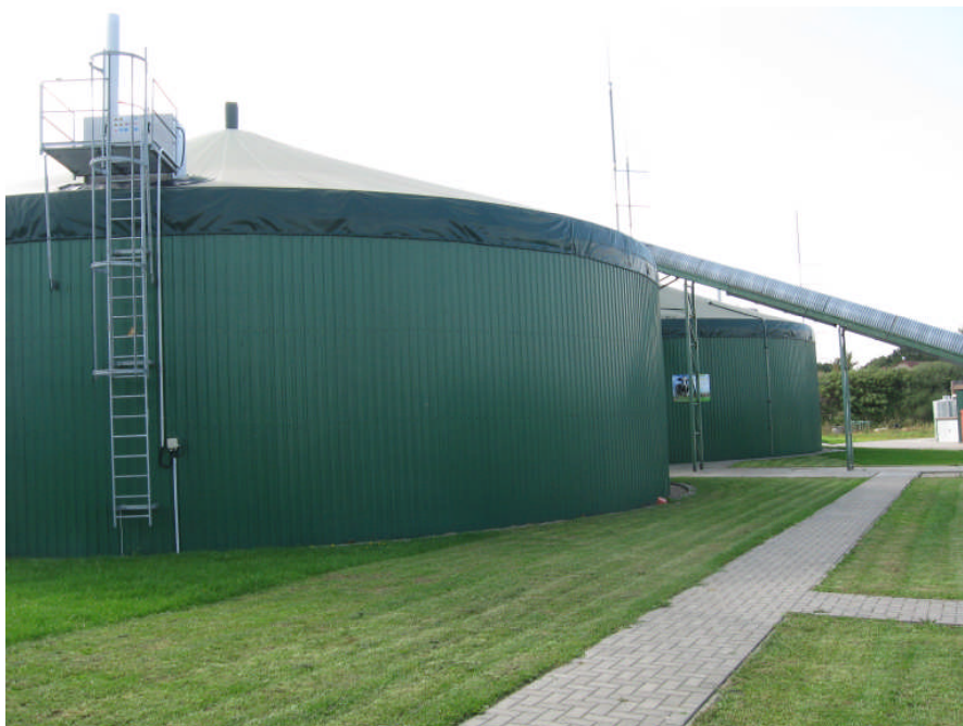
Picture 1 The biogas plant Tangeln
